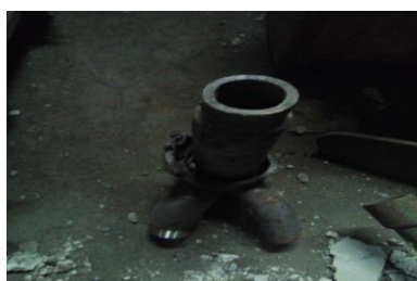
Gambar 9. Kerusakan middle part RCB
